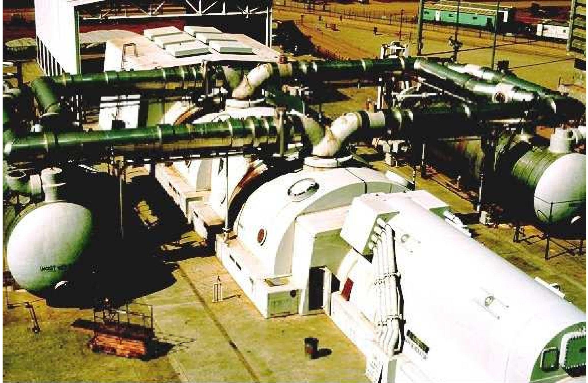
Overview of a steam turbine and main generator for a nuclear steam power station. (Courtesy of Carolina Power and Light Company)
